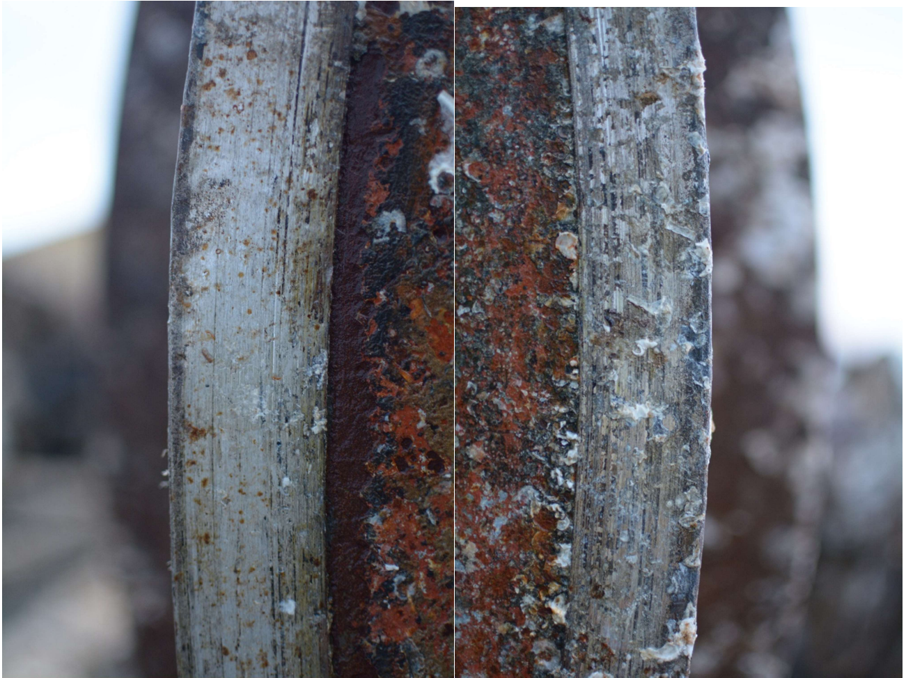
Figure 42 - Large version tower flange 9 and 3 o'clock positions
